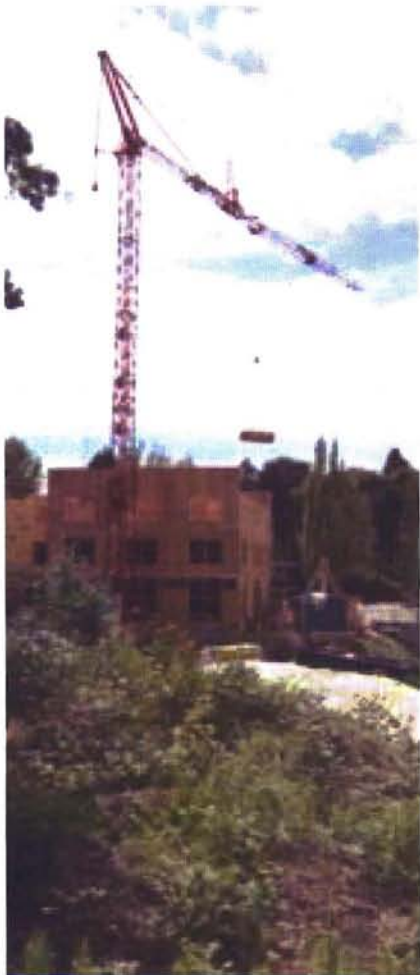
A Potain Igo T 70 self-erecting crane works on a multi-residence building in Seattle, Washington. The crane is being rented by general contractor RAFN Company from Coast Crane Company
