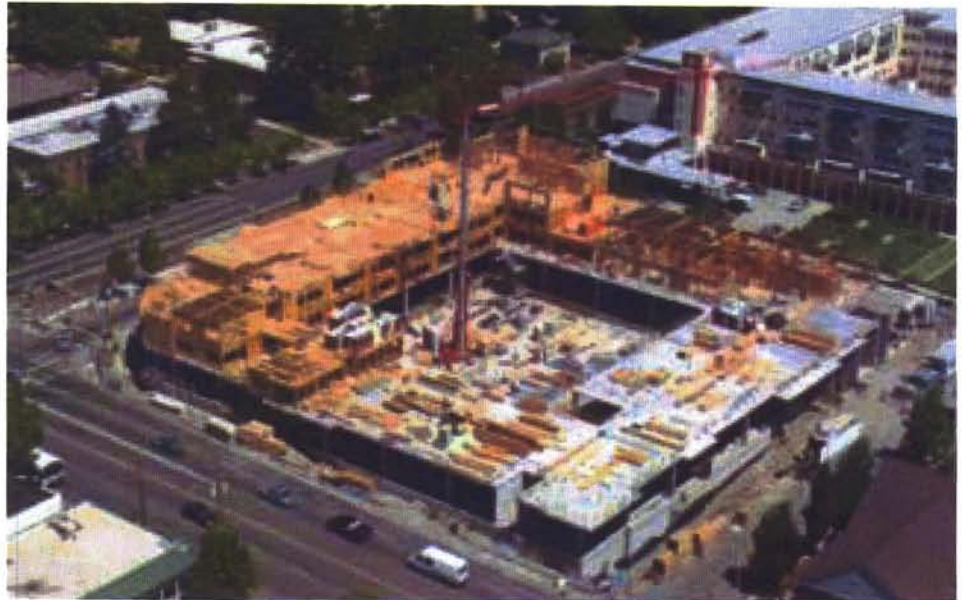
This Potain HDT 80 self-erecting crane is building a five-story, 142-unit assisted living retirement complex in Portland, Oregon. The crane was rented to general contractor Yorke & Curtis by Coast Crane Company
